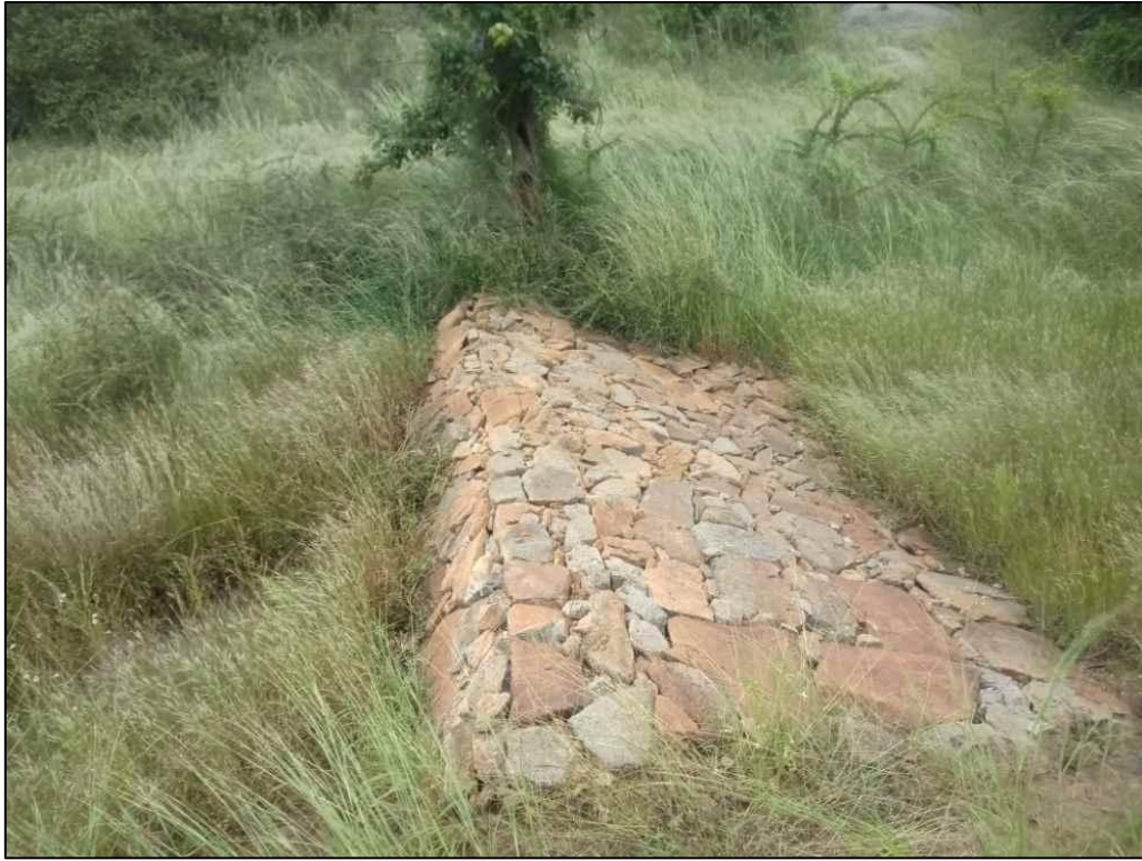
Photo 7: Gully checks, Gudekote range, Ballari division, Ballari circle Good quality work
