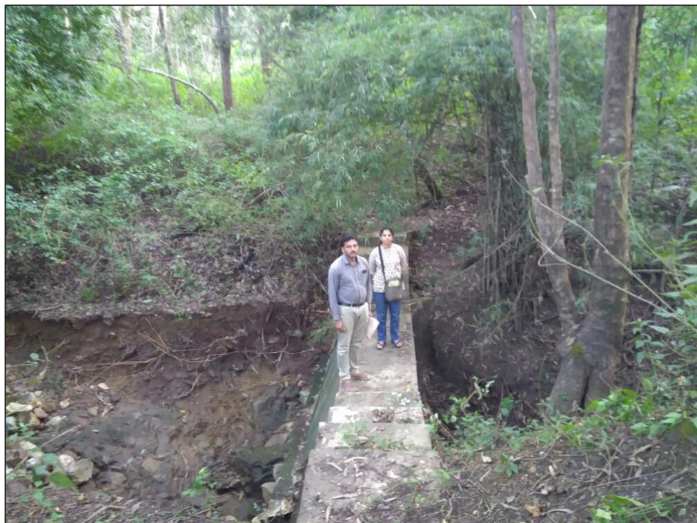
Photo 23: Check dam, Lakkavalli range, Bhadravathi division, Shivamogga circle Filled with vegetation and partially breached
